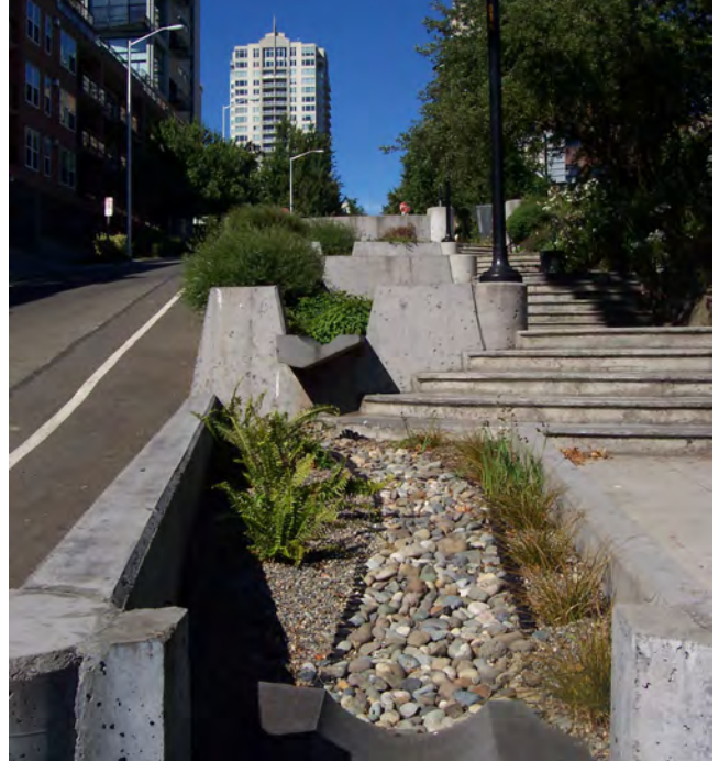
FIG. 4-11 This artful stormwater conveyance system is part of a community garden in Seattle’s Belltown neighborhood.
