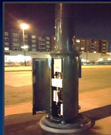
Equipment Inside of Pole Base
