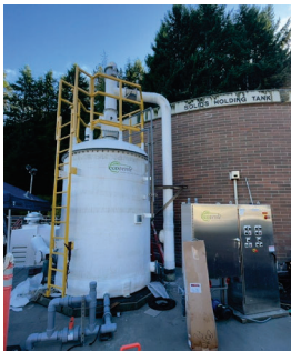
NETP Solids Holding Tank Bioscrubber Project $1.5M
