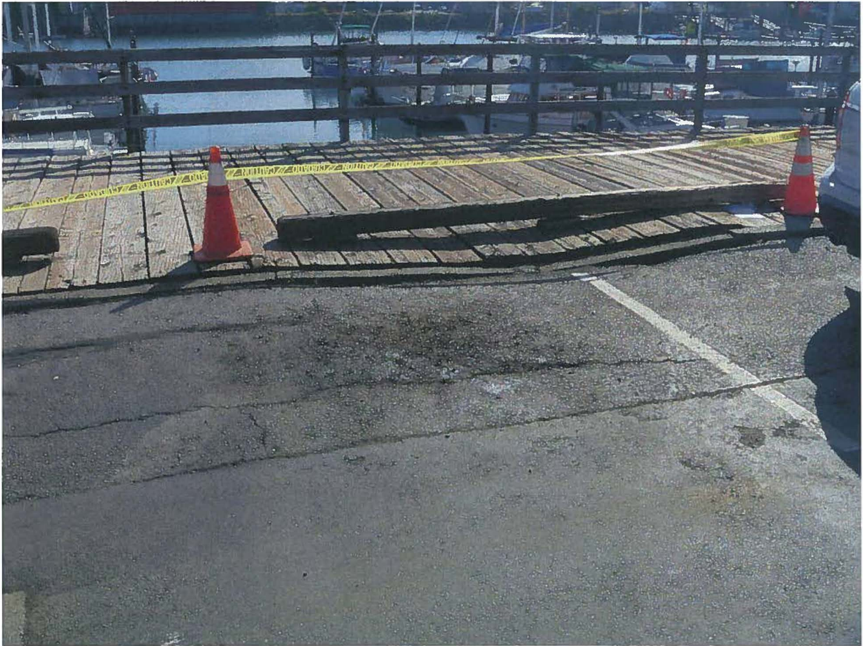
This photo shows the failing wood deck and adjacent asphalt parking area.
