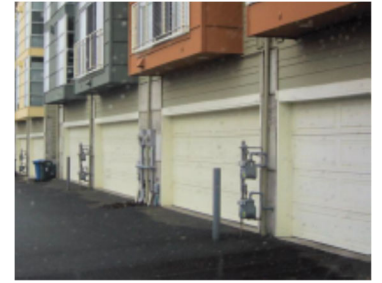
Exposed utility meters like this will not be allowed where visible from common open spaces, streets or pedestrian areas.
