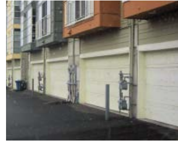
Exposed utility meters like this will not be allowed where visible from common open spaces, streets or pedestrian areas.
