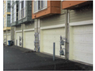
Exposed utility meters like this will not be allowed where visible from common open spaces, streets or pedestrian areas.
